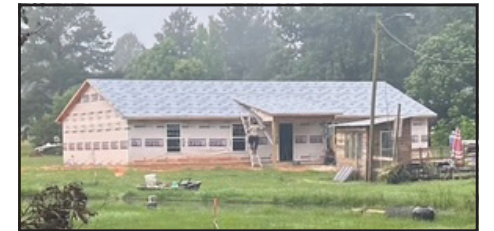
The community has been very generous and donated all materials and labor for the construction of the foundation.
