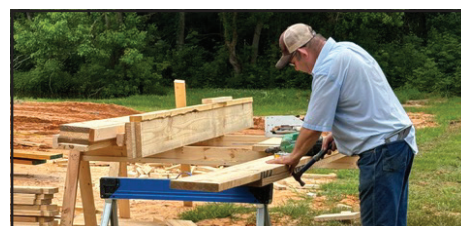
Generous community donations include workmanship for electrical, sheetrock, plumbing, insulation, HVAC, and cabinets.
